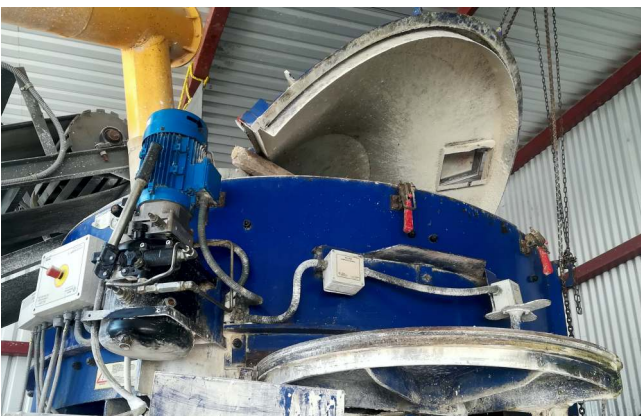
Mixer installed for the production of precast.
