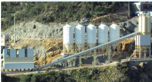
Transfer system and dense phase pneumatic transport for cement, filler and ash.
